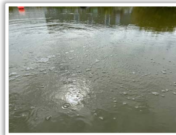
Nanobubbler aeration (Moleaer Clear 150).
